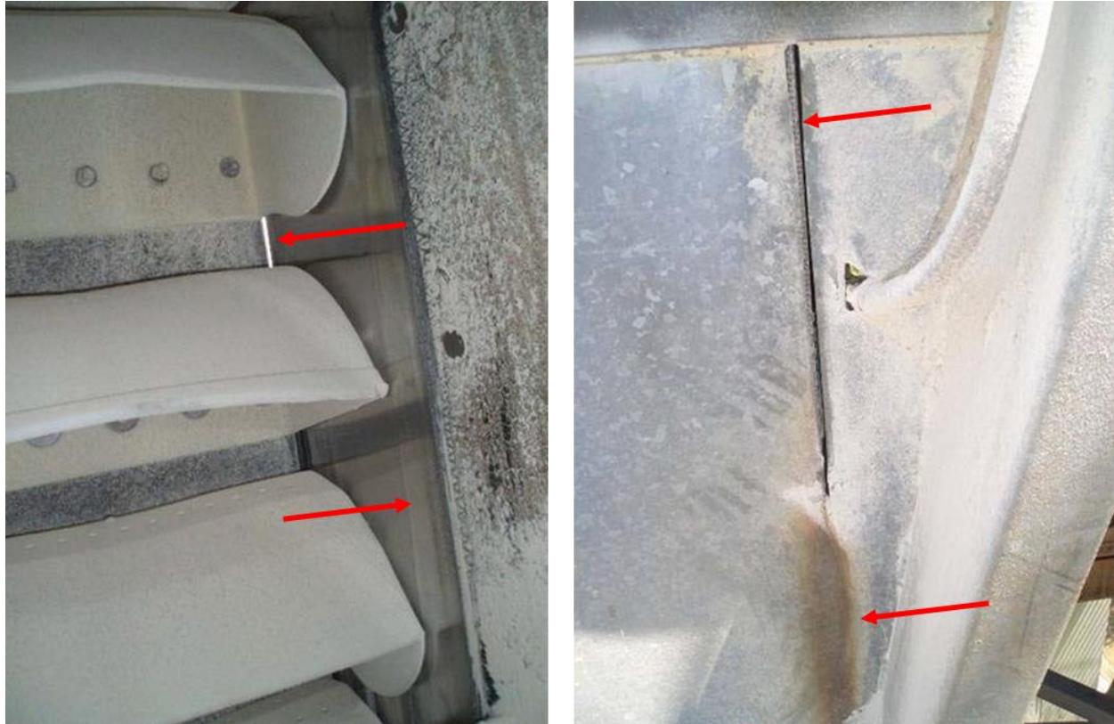
Figure 16: Inside elevator (left) and outside elevator (right) showing discoloration and slits in steel casing from the effects of friction and wear due to severe belt misalignment. (Photographs courtesy of 4B Components, Ltd)
