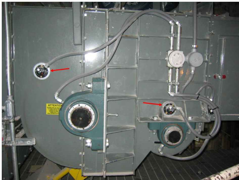
Figure 20: Force activated belt misalignment switches installed on an enclosed belt conveyor. (Photograph courtesy of 4B Components, Ltd)
