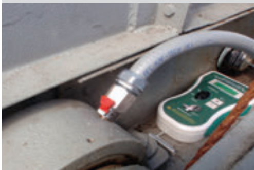
ADB Sensor Installed on Conveyor Bearing
