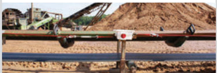
Pullswitch installed on open belt conveyor
