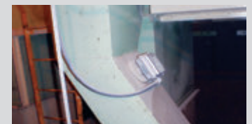
Auto-Set™ Flush Probe Installed on Belt Conveyor Discharge
