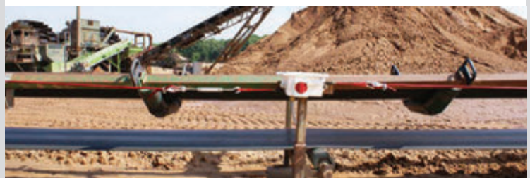
Pullswitch installed on open belt conveyor
