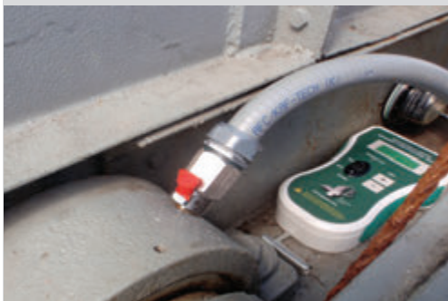
ADB Sensor Installed on Conveyor Bearing
