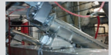
Auto-Set™ Flush Probe Installed on Screw Conveyor Discharge
