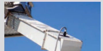
Bin switch Installed on Bucket Elevator Spouting (with SMP, BAS & conduit adapter)
