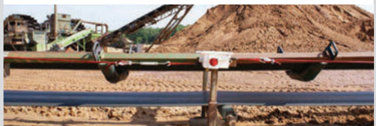
Pullswitch installed on open belt conveyor
